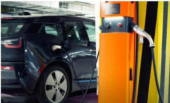
EV Charging Station
